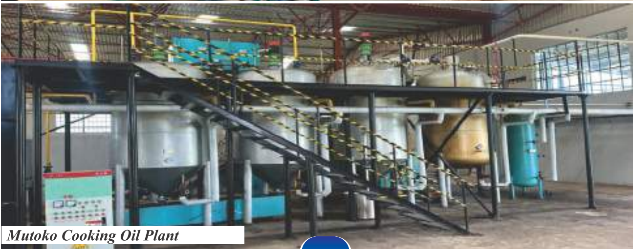
Mutoko Biodiesel Plant
