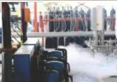
Verify Engineering Medical Oxygen Plant
